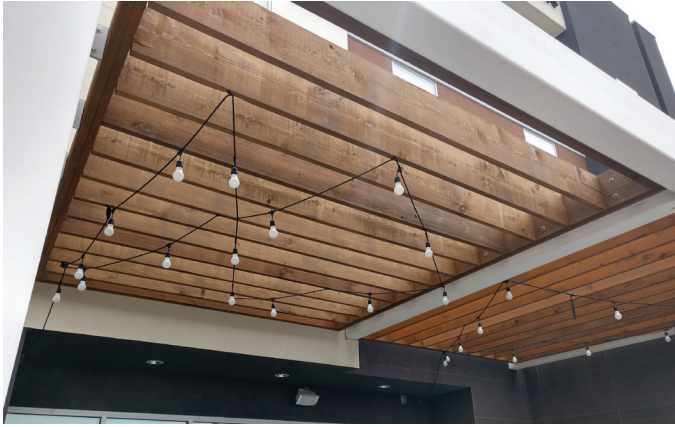
Exterior Fire-X® is often used in weather-exposed applications like this hotel pergola in Denver, CO.
