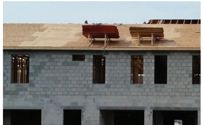
Pyro-Guard® plywood used four feet on each side of a wall to eliminate parapets. St. Petersburg, FL.
